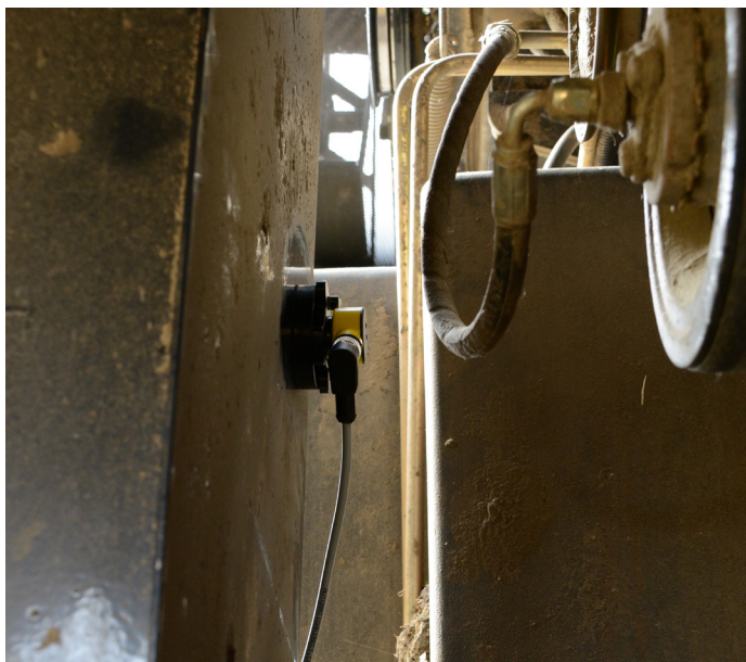
Back of elevator
